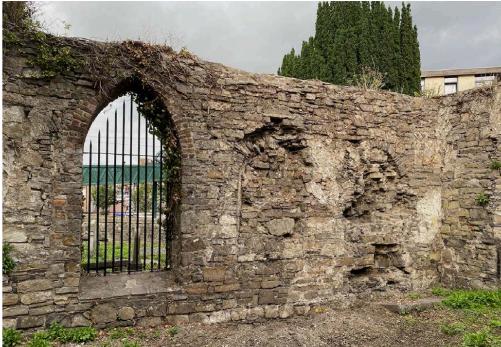
50. View of exposed north chancel wall showing former openings in vulnerable condition.
