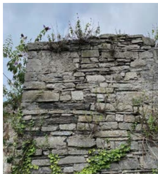
41. Loose stone at high level to nave.
