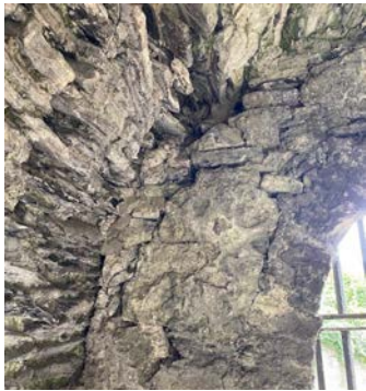
40. Voids and cracks to stone vault to entrance porch
