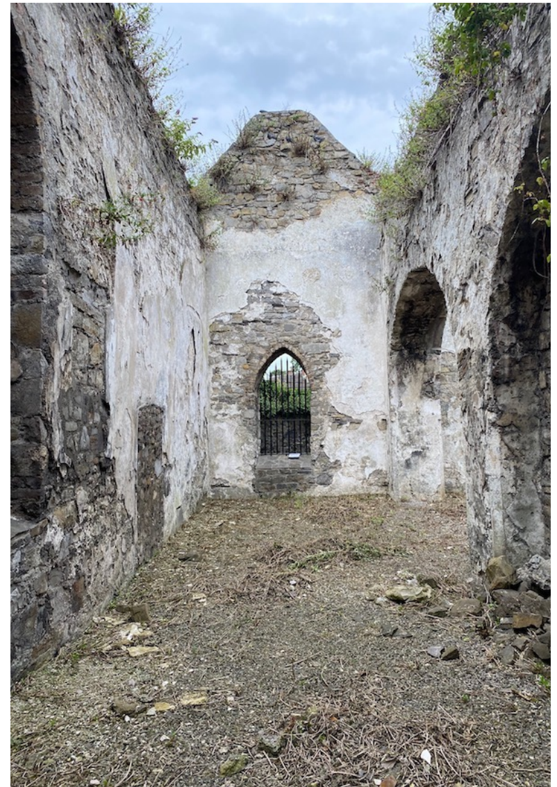
49. View looking west in side chapel. Note fallen plaster on floor.
