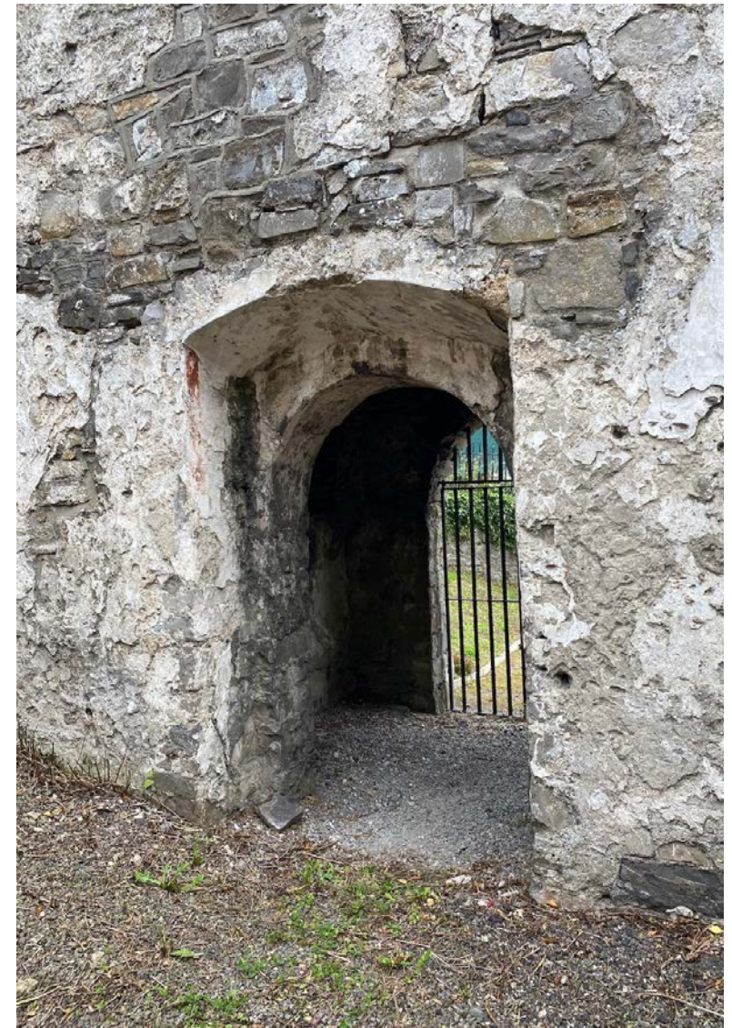
54. View of main entrance door in nave. Note red pigmented plaster to reveal.
