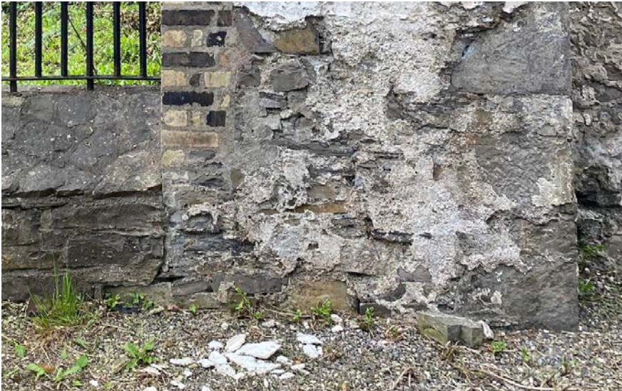
89. Broken recumbent slabs close to entrance porch and bridge in background.
