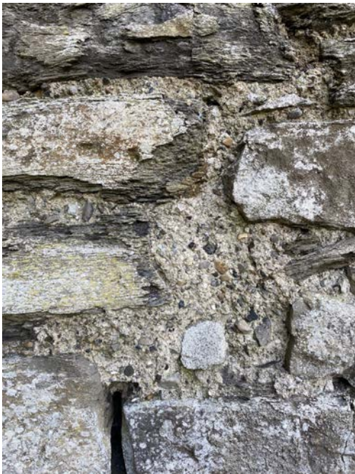
55. Lime mortar and eroding Calp.
