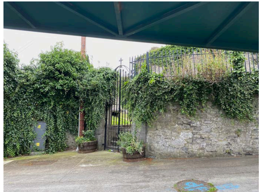
14. View of entrance gate from underneath bridge showing extent of ivy.
