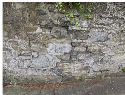
18. Large cracks and bulging to boundary wall along footpath.
