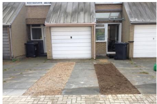
Image: Driveway with SuDS incorporated
