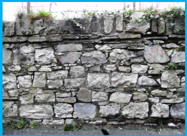
Views of section of calp limestone wall which forms western boundary of ACA between railway line and Great Western Square/Great Western Villas
